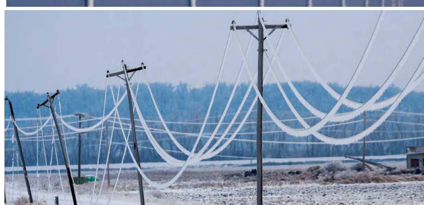
Power Lines & Heating Systems
